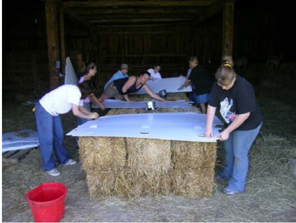
Indraloka Animal Sanctuary volunteers prefold Yurt wall panels on bails of straw that will later be used to insulate the structures.
