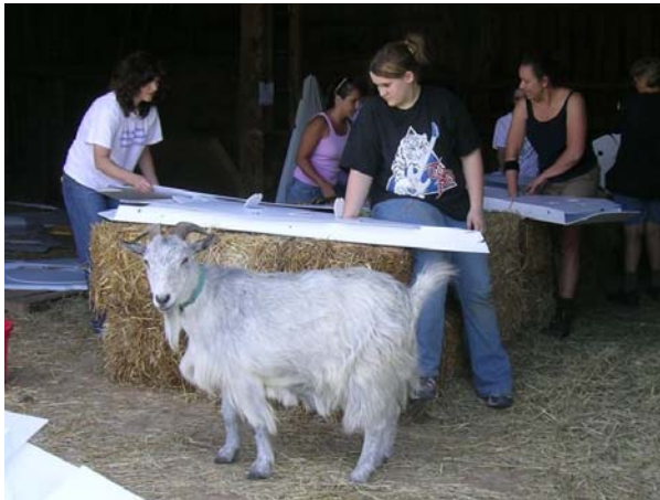
With all the panel parts creases prefolded, volunteers fold the pre-cut flat sheets into three-inch thick (7.62 cm) wall, roof, window and door parts.
