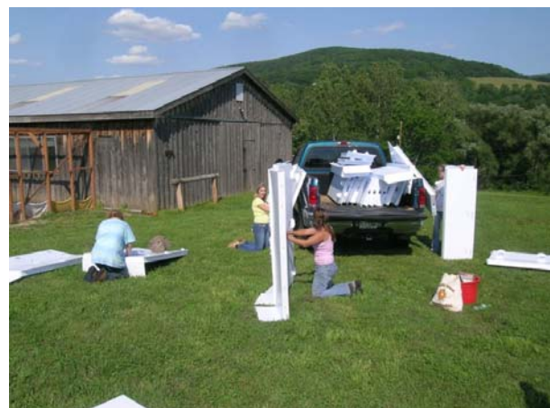
Volunteers begin assembling the Yurt walls by bolting preassembled wall panels together.
